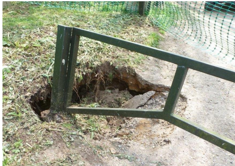
Figure 3: Sink hole at the Vale of Health.
